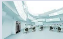
Distributed control systems
